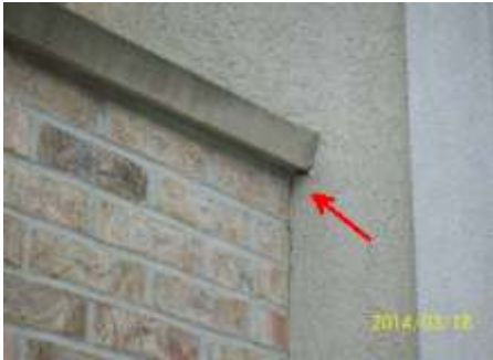
EIFS / Chimney junctions should be sealed.
