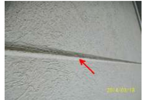
Architectural groove is not a proper expansion joint.
