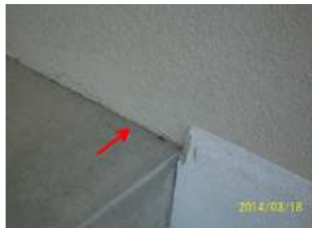
Recommend sealing the front stoop EIFS Junction.
