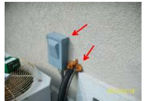
Unsealed or improperly sealed utilities.
