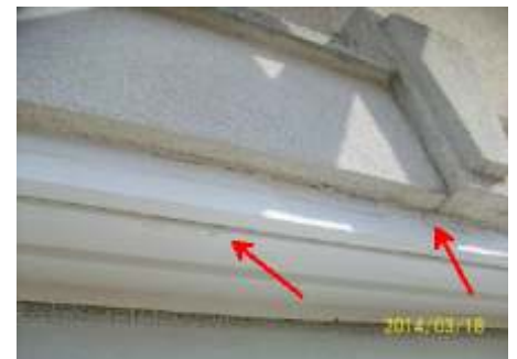
Evidence of moisture weeping from garage door header. Rotted wood.
