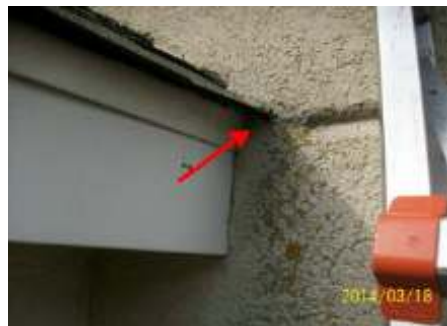
Missing kickout flashing.
