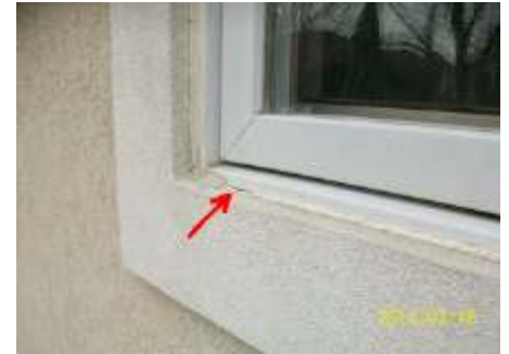
Gaps in old window sealants.
