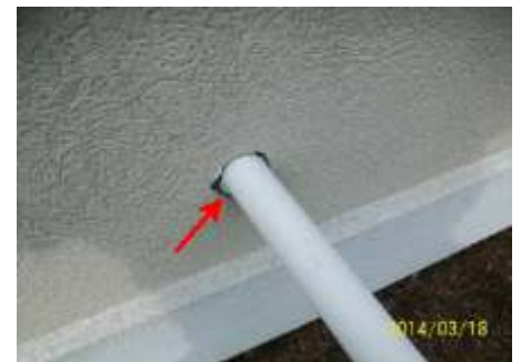
Piping penetrations should be sealed.
