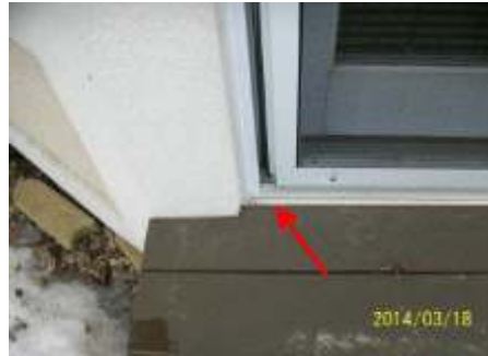
Unable to test under rear door due to wooden step.
