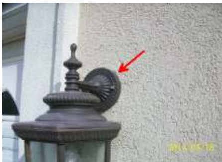
Light fixtures should be sealed.
