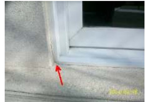
Minimal use of sealant has failed.
