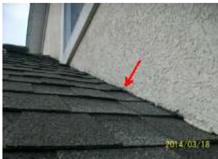
Improper roof line termination.
