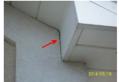
Soffit & Fascia should be sealed.
